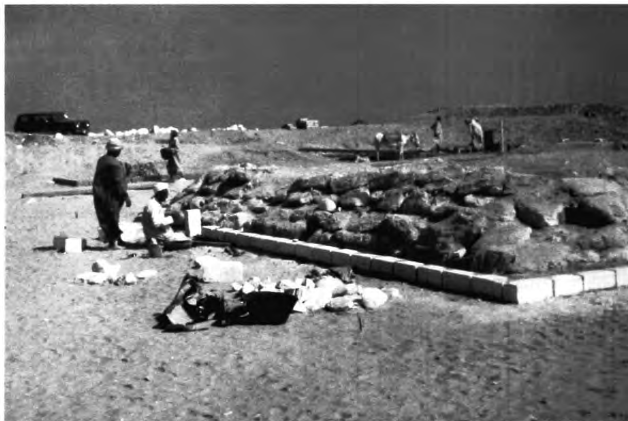
ARCHAEOLOGY. Excavations of Dieter Arnold at el-Lisht, 1989. Repair work on the western side of Imhotep's mastaba . (Courtesy Dieter Arnold)
